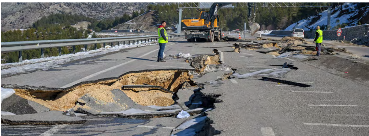
The roads that collapsed due to the intensity of the earthquake are being repaired. Efforts continue to mend the roads that collapsed due to the severity of the earthquake in Adiyaman, one of the provinces most affected by the earthquake centred in Kahramanmaraş. Many sections of the Adiyaman-Malatya highway became completely unusable, and retaining walls collapsed during the 7.7 and 7.6 magnitude earthquakes, whose epicentre was Kahramanmaraş and affected 10 provinces. The General Directorate of Highways initiated efforts to repair the collapsed highway to facilitate smoother transportation of aid to the city. (Özkan Bilgin - Anadolu Agency)
